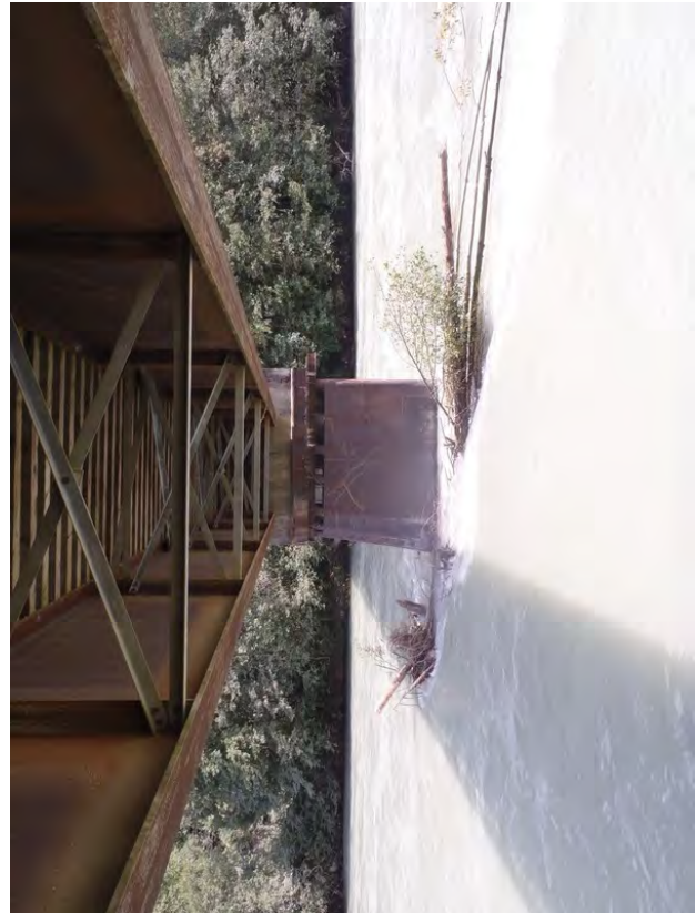
Figure 20: Pier 2 right end face - Note debris jam upstream.
