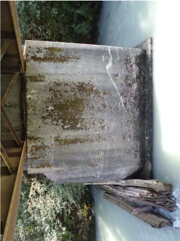
Figure 18: Pier 1 right end face - Note debris jam upstream.
