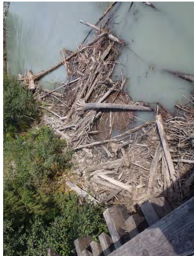
Figure 31: Debris jam at right end upstream.
