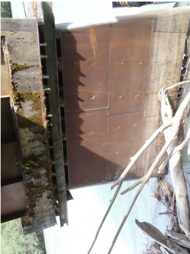
Figure 21: Pier 3 right end face - Note debris jam upstream.
