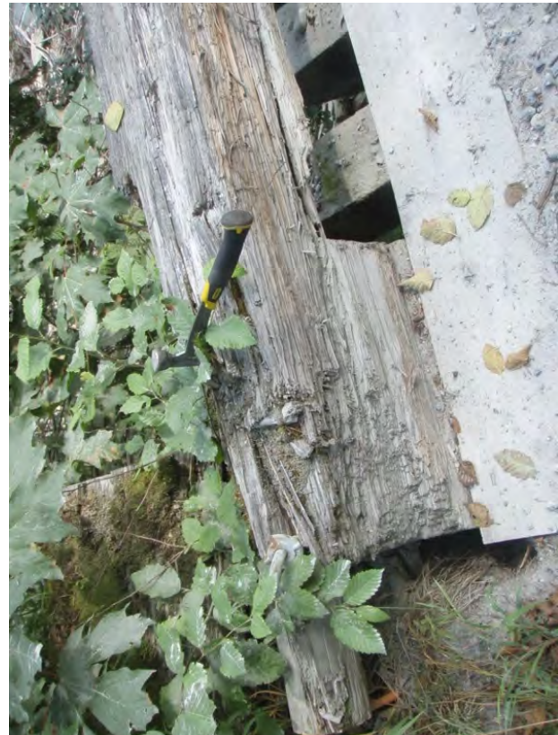
Figure 11: Typical rot in curb rail - Span 4 upstream right corner shown.
