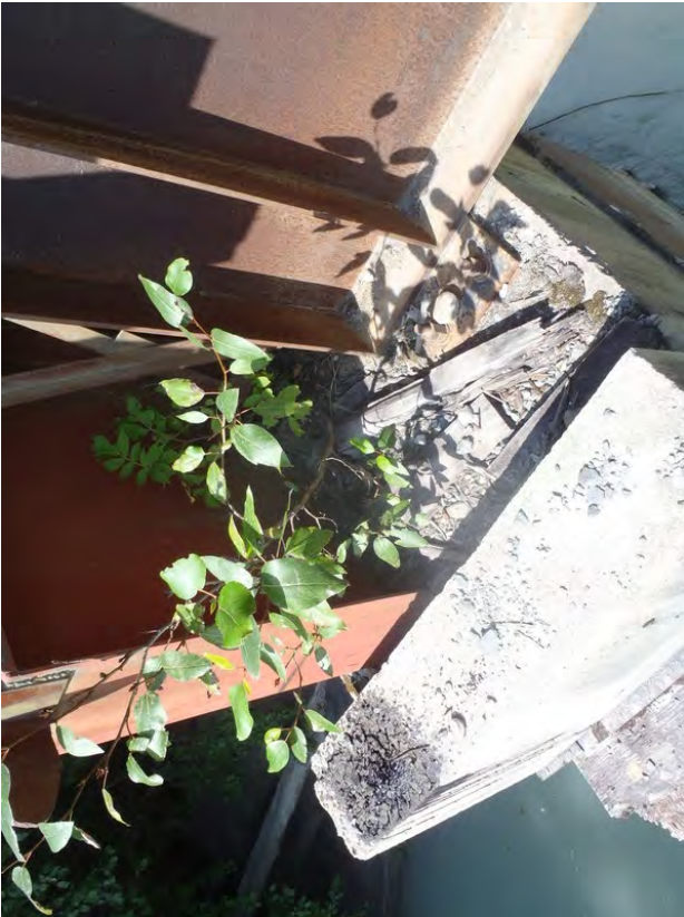
Figure 26: Pier 2 concrete cap - Note debris and vegetation.
