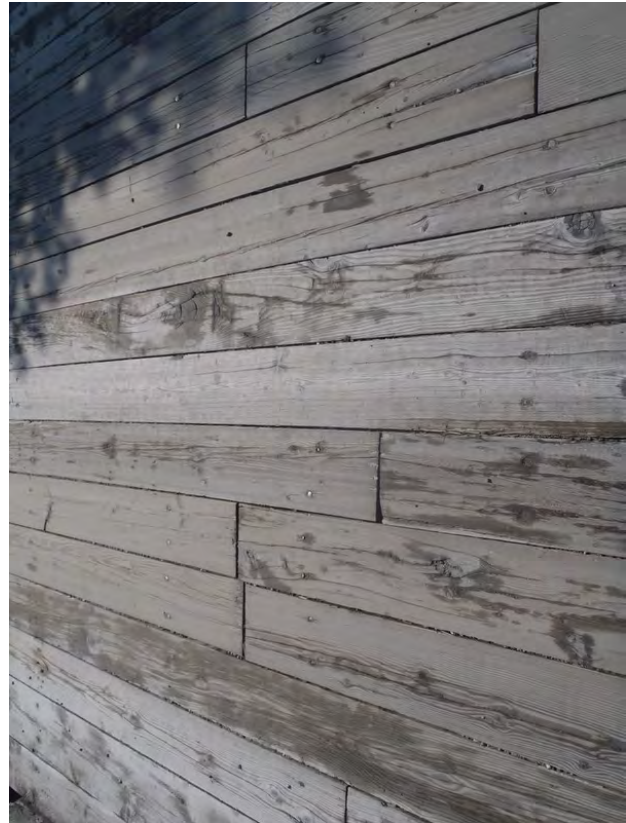
Figure 8: General deck condition - Note substandard nail spacing.
