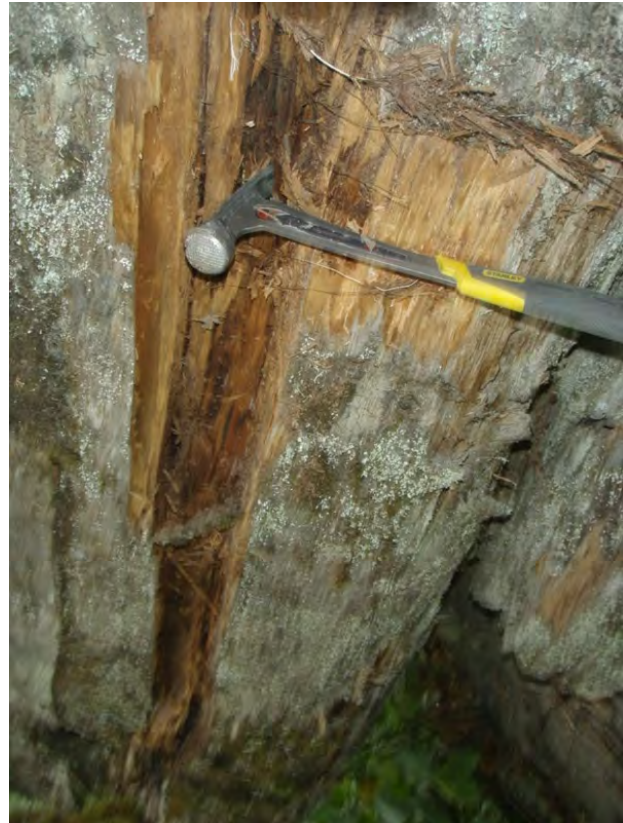
Figure 16: Outer heartwood rot in right abutment ballast wall.
