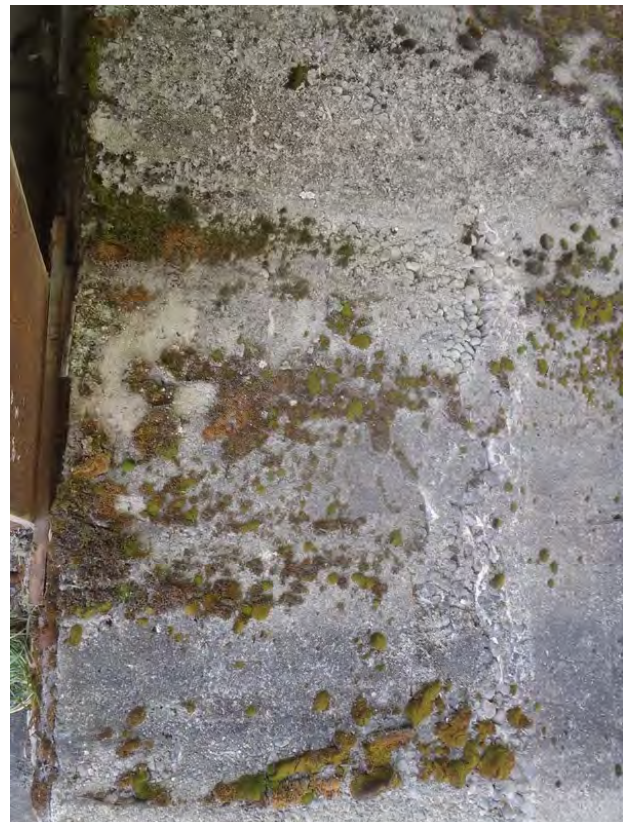
Figure 23: Right face of Pier 1 concrete wall - Note exposed aggregate and poor consolidation.
