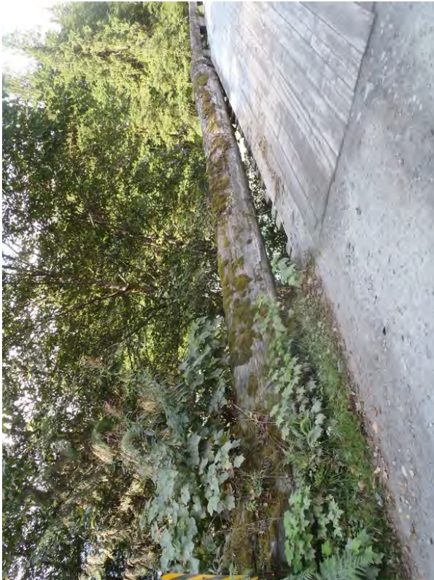
Figure 10: Span 1 downstream curb log - Note gap between log and edge of deck.
