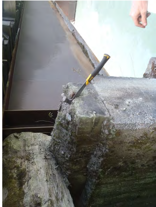
Figure 24: Pier 1 Span 1 timber sill - Note rot in end of sill.
